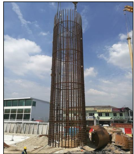
Steel reinforced cage for a 2.8-metre diameter bore for an infrastructure project
